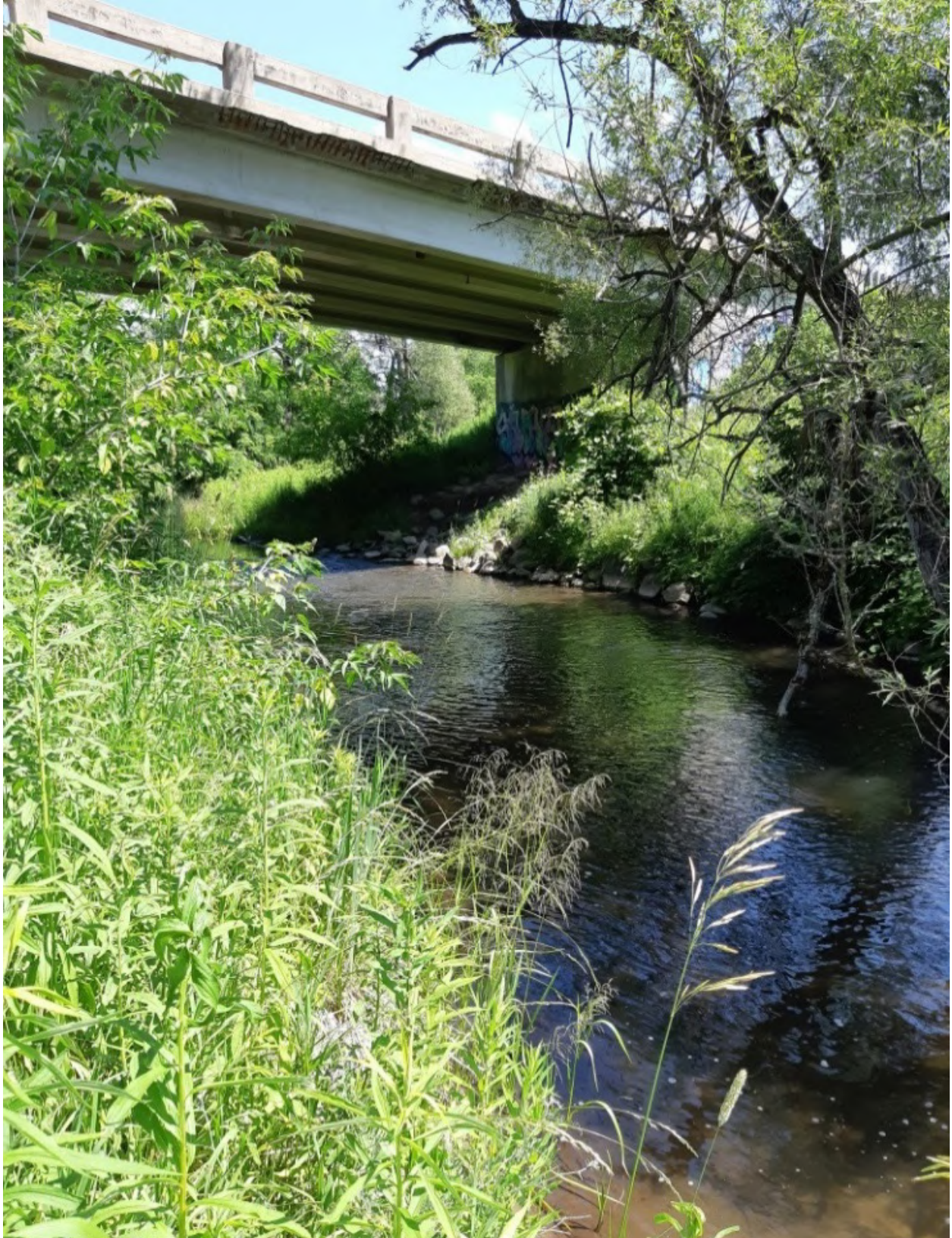
Looking at a riparian crossing from stream level. Clearance is adequate but requires a level terrestrial pathway at grade or slightly higher than water levels for wildlife passage.
