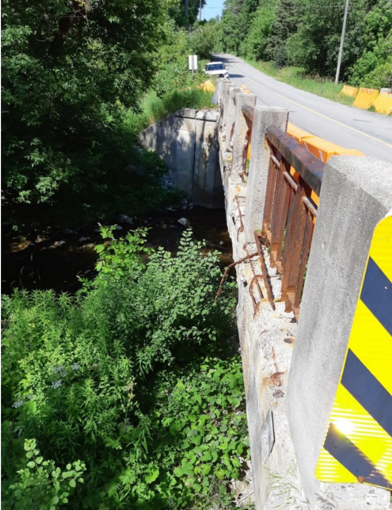
Site 1: 7 th Concession and Sideline 32 with wing walls that are ideal for tying in wildlife funnel barrier to the structure.
